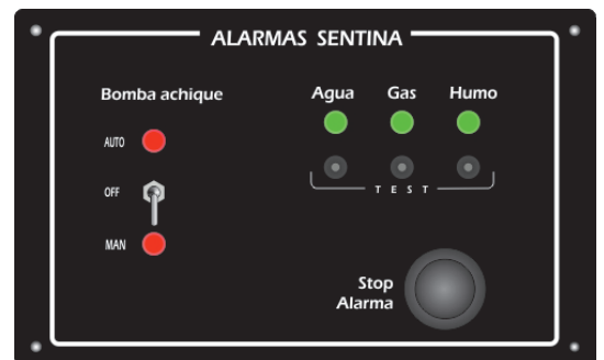
Panel in Manual mode, Pump working
